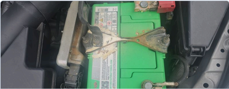
Plate 4: Battery & ECM Mounting Proximity Corroded tie-down bracket resting loose across battery. Check ECM casing & wire harness directly adjacent.
